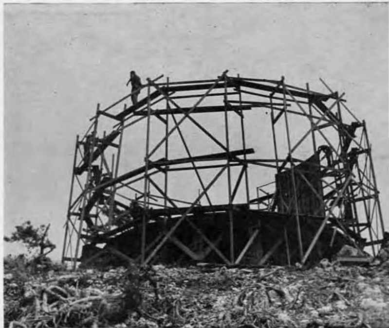
Our 126,000-gallon water tank perched on the highest height in camp.
