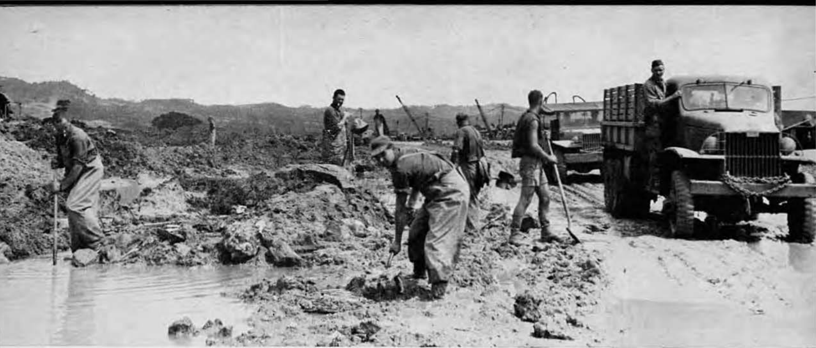
Three shifts shovelled to drain water and fill holes on the supply road to the front lines.
