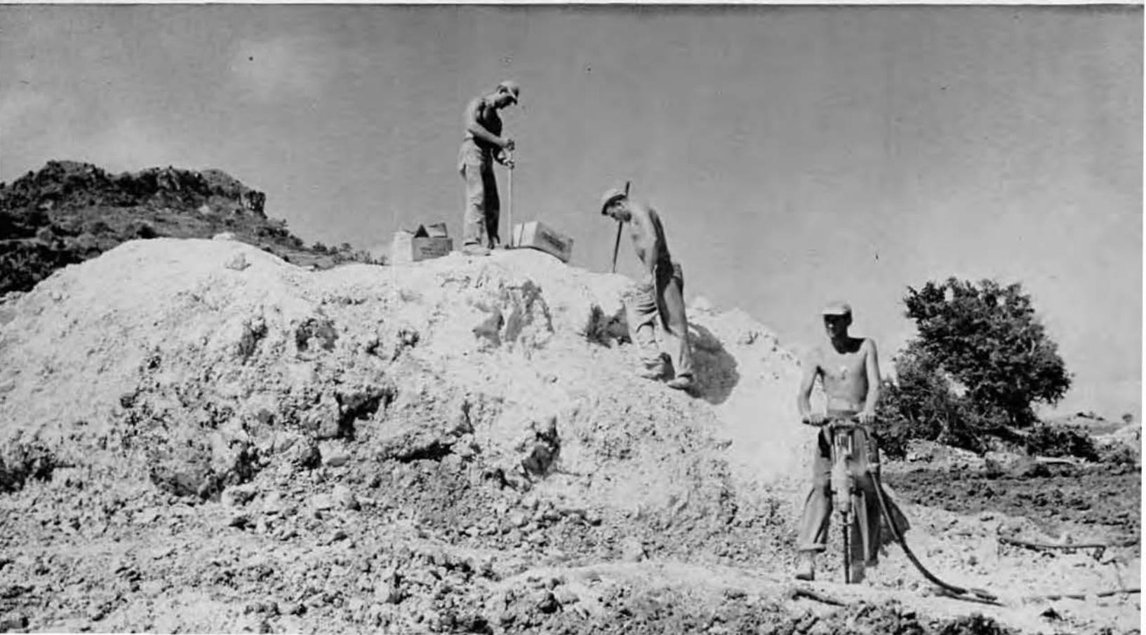
Macht, Horbach and Footer drilled holes for blasting away rock in the road right-of-way
