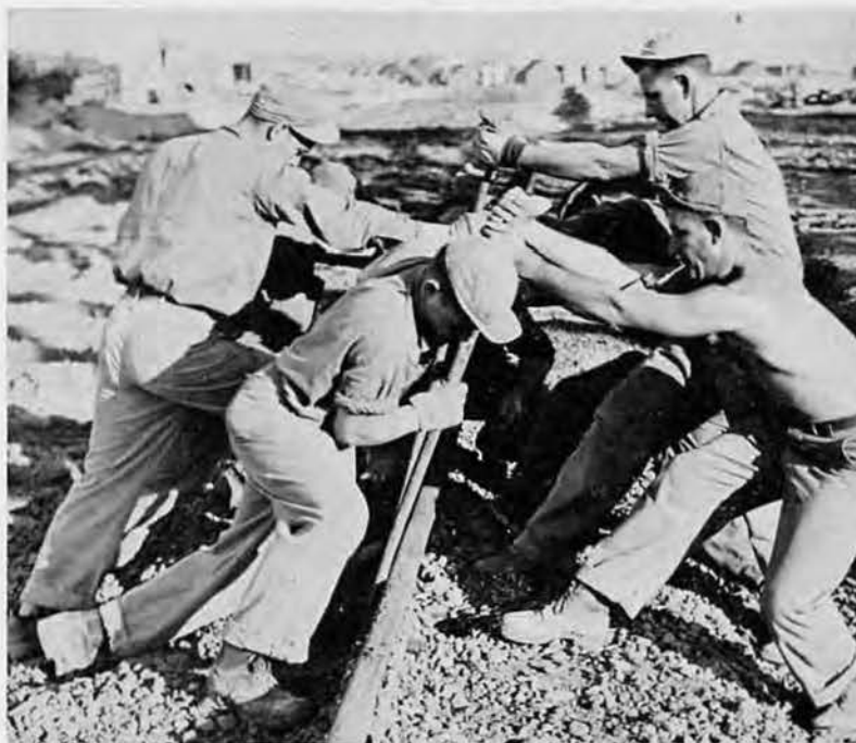
Below: "Elbow-grease" aligned the iron-rail runways Bottom: The runways were solid for 60-ton loads
