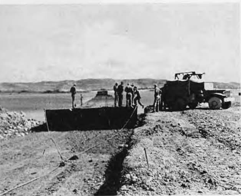
One end of the pontoon assembly was pulled ashore by a "cat"
