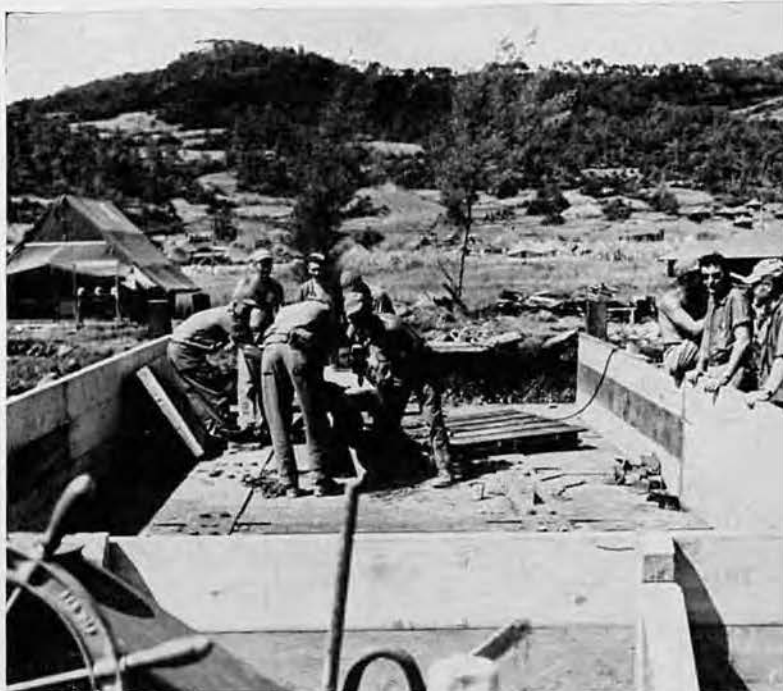
Top: Seventeen acres were cleared and graded for the 17th Seabee Regiment dump.
