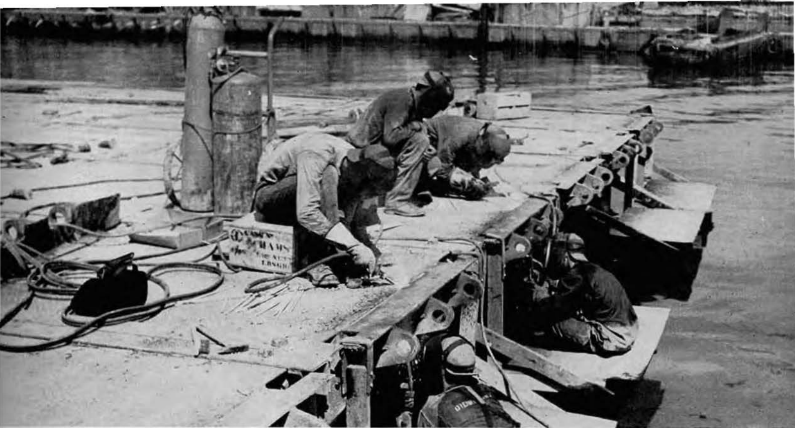
The pontoon sections were held together by hinges which were welded to the sides
