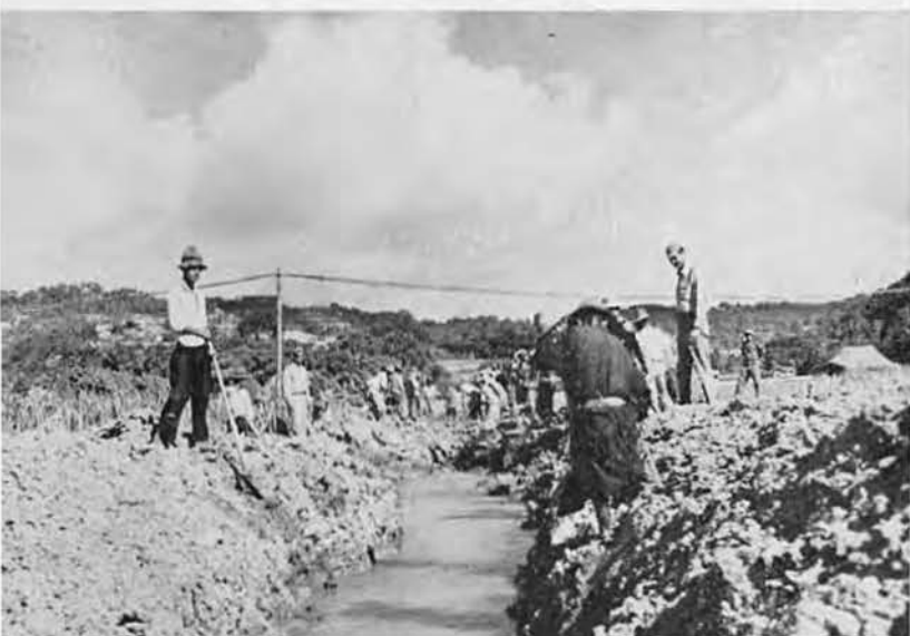
Okinawan labor crews, usually barefoot, helped dig us out of the mud.
