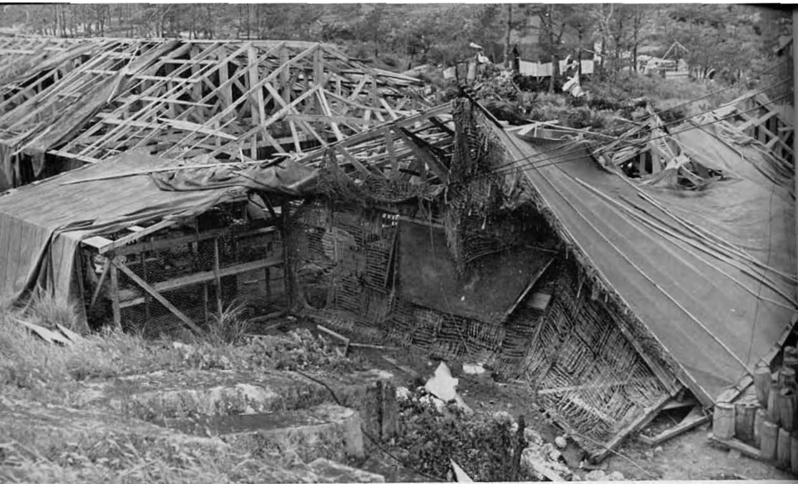
The carpentry shop was smashed, as were the heavy equipment repair and transportation shops
